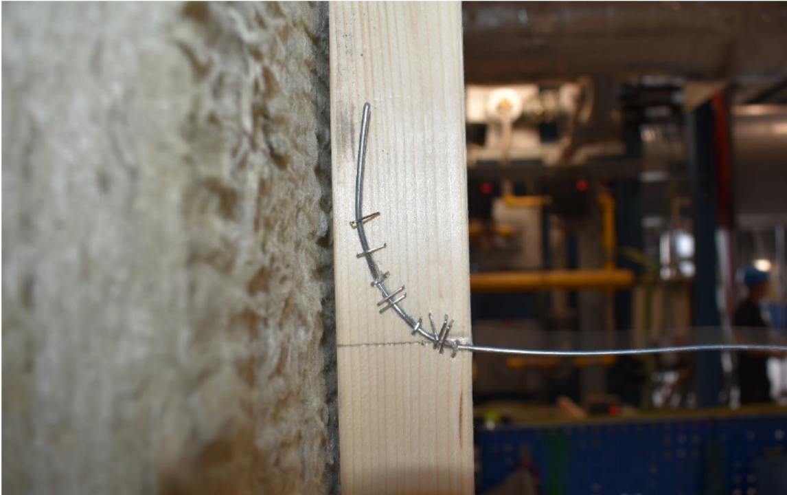
Photo No. 3 Wire fastened to stud.
