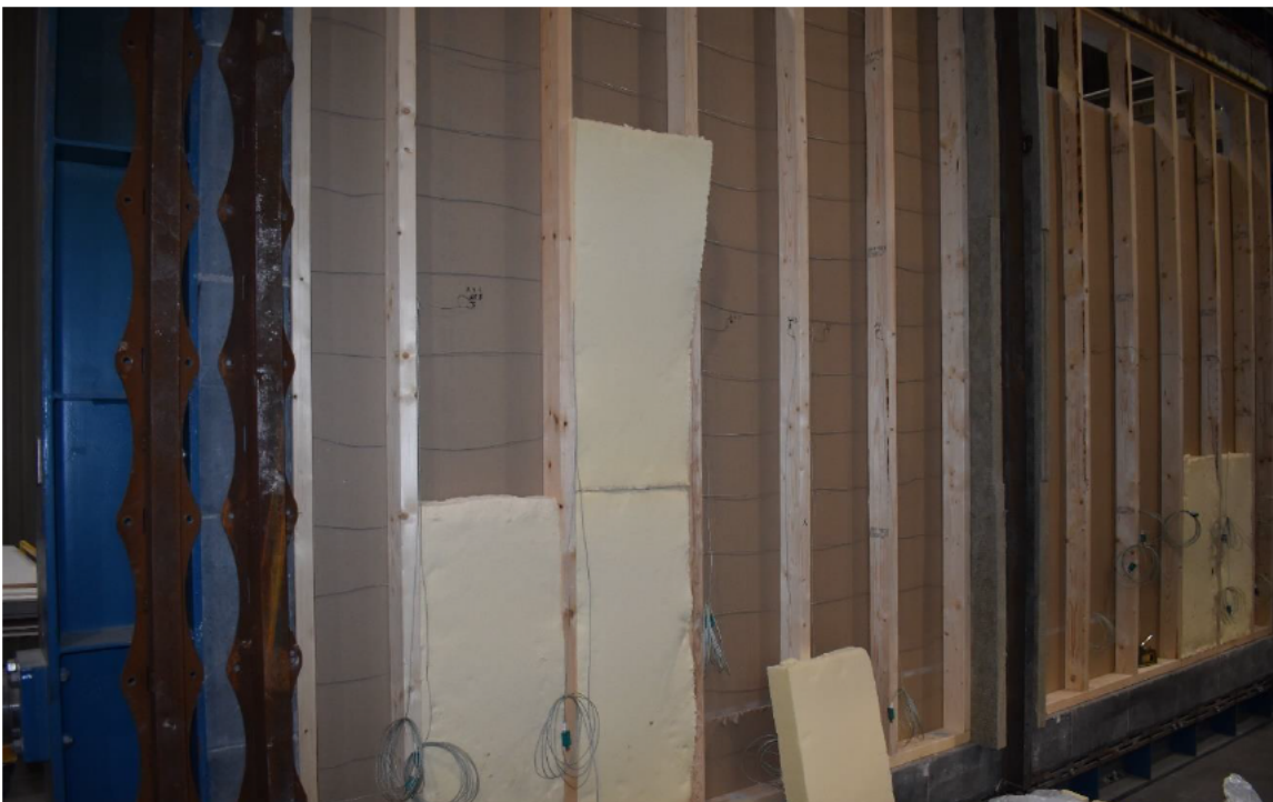
Photo No. 6 Insulation slabs being mounted on the side with the wire.
