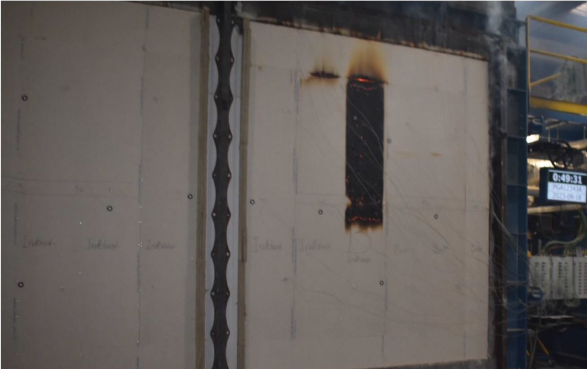
Photo No. 19 Gypsum board with heavy discoloration. On side B
