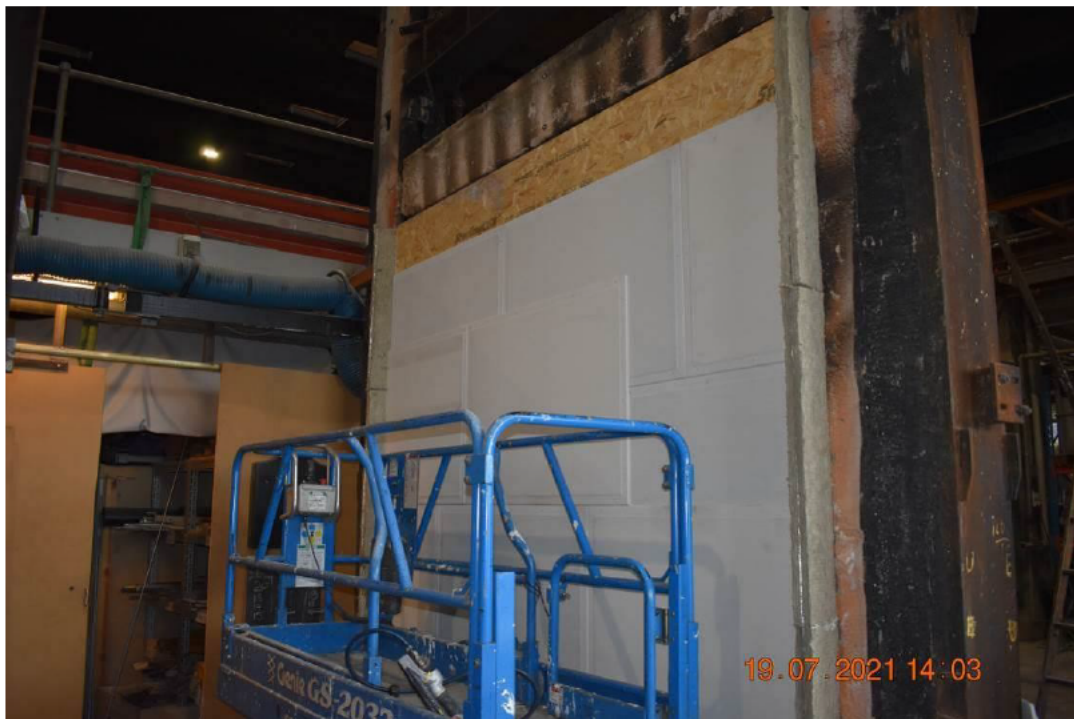
Photo No. 4 Both layers of fibre gypsum boards mounted to the OSB-3 board.
