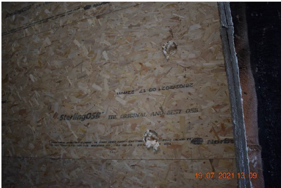
Photo No. 2 Holes in the wall showing the wood fibre insulation between wooden studs.
