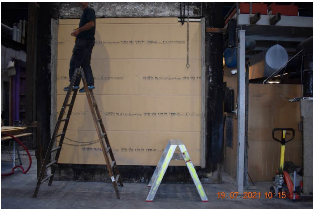
Photo No. 6 Layer of wood fibre board mounted to studs on the exposed side.
